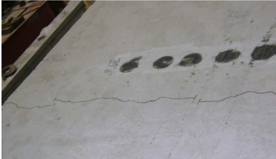
Figure 65: Shrinkage Crack Extending Across Top of Deck
