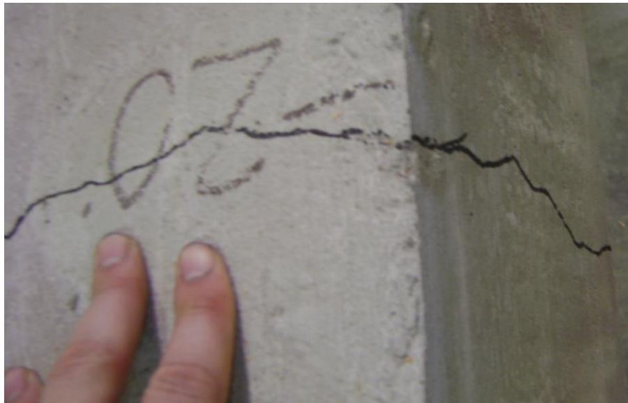
Figure 64: Shrinkage Crack Beginning on Edge Continuing on Top of Deck
